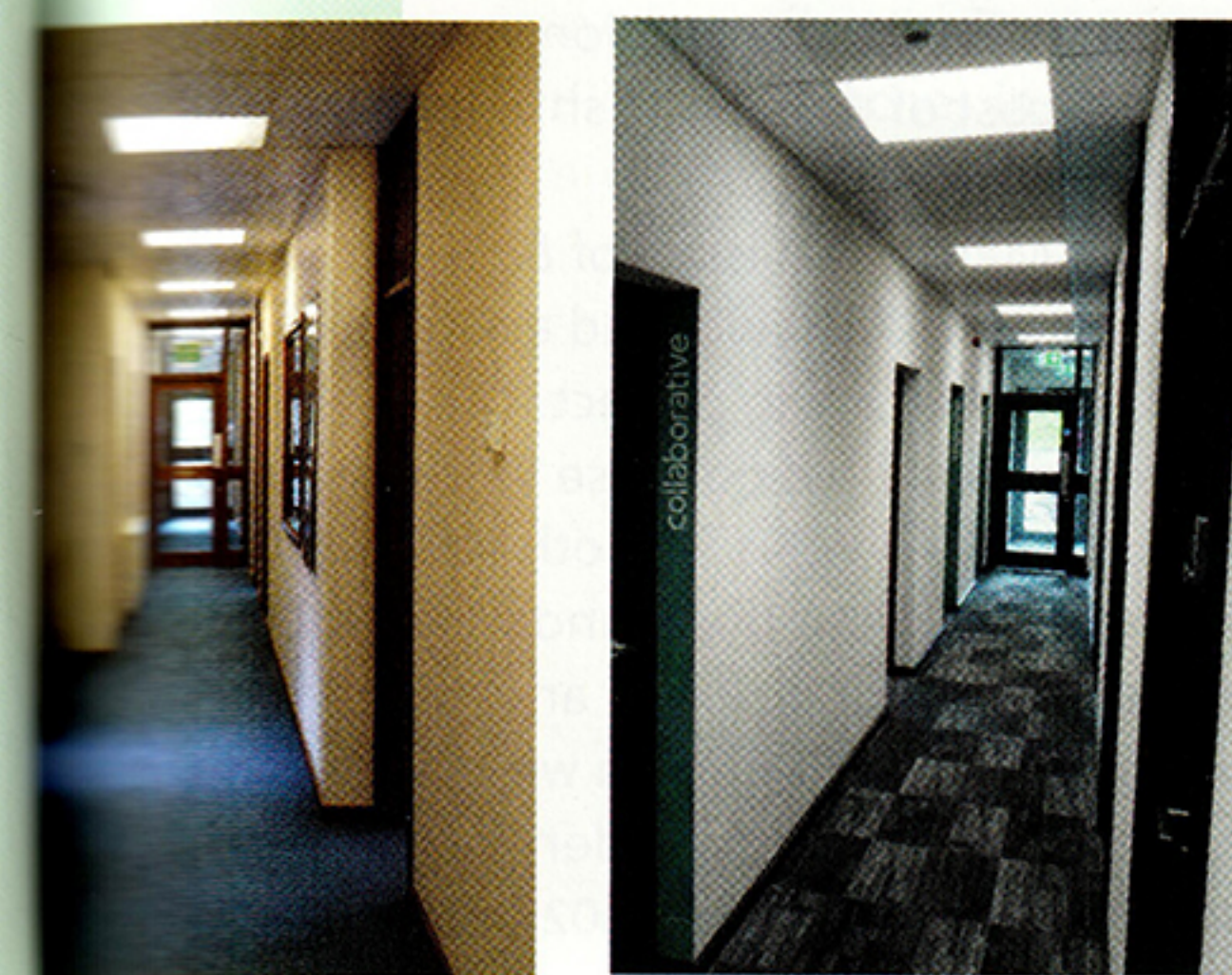
▲ The hardwood for the internal doors, frames, skirtings and architraves was retained and refurbished wherever possible rather than using new door sets
