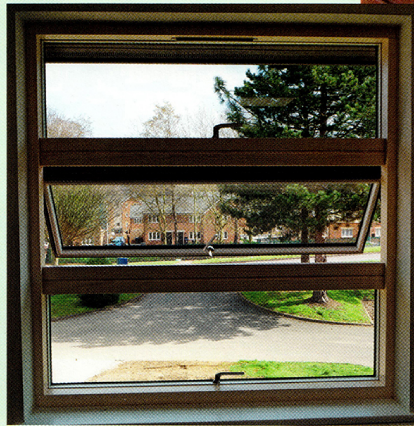
▲ Double-glazed windows and thermally insulated spandrel panels replace the old uninsulated ones
