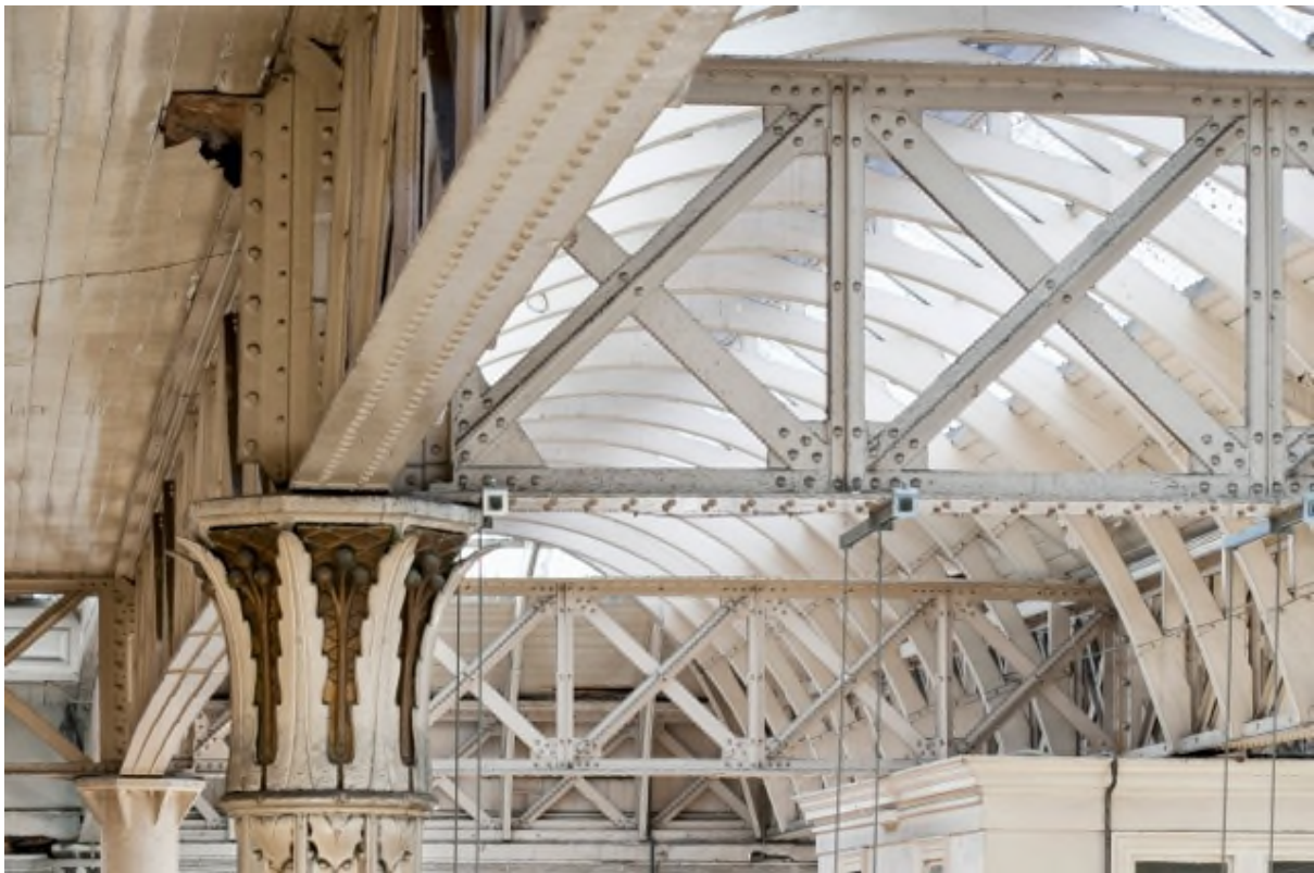
01 - The 'phoenix columns', an ornate and innovative detail supporting the light and airy roof
